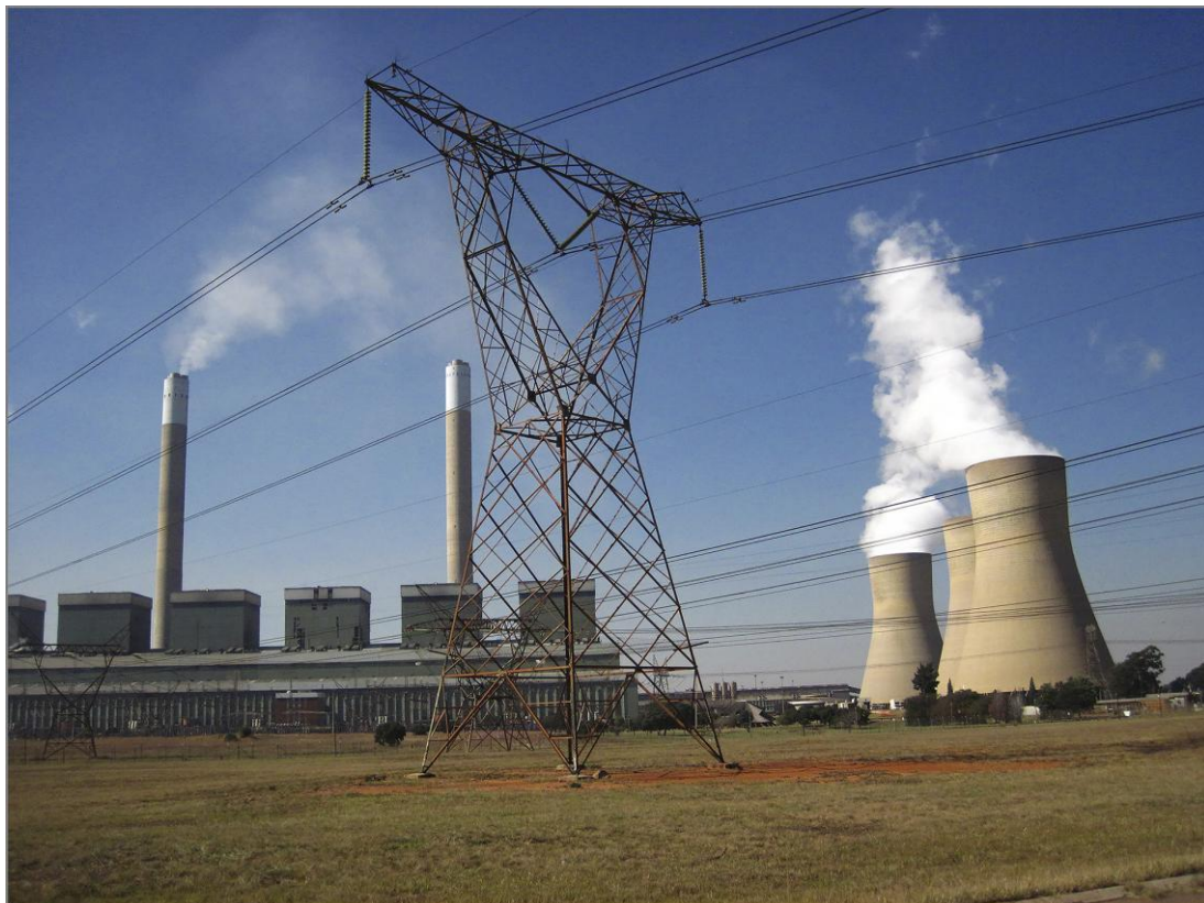
Figure 8: The outgoing lines exiting to the south-west across cut grassland within and outside the Duvha security compound.
